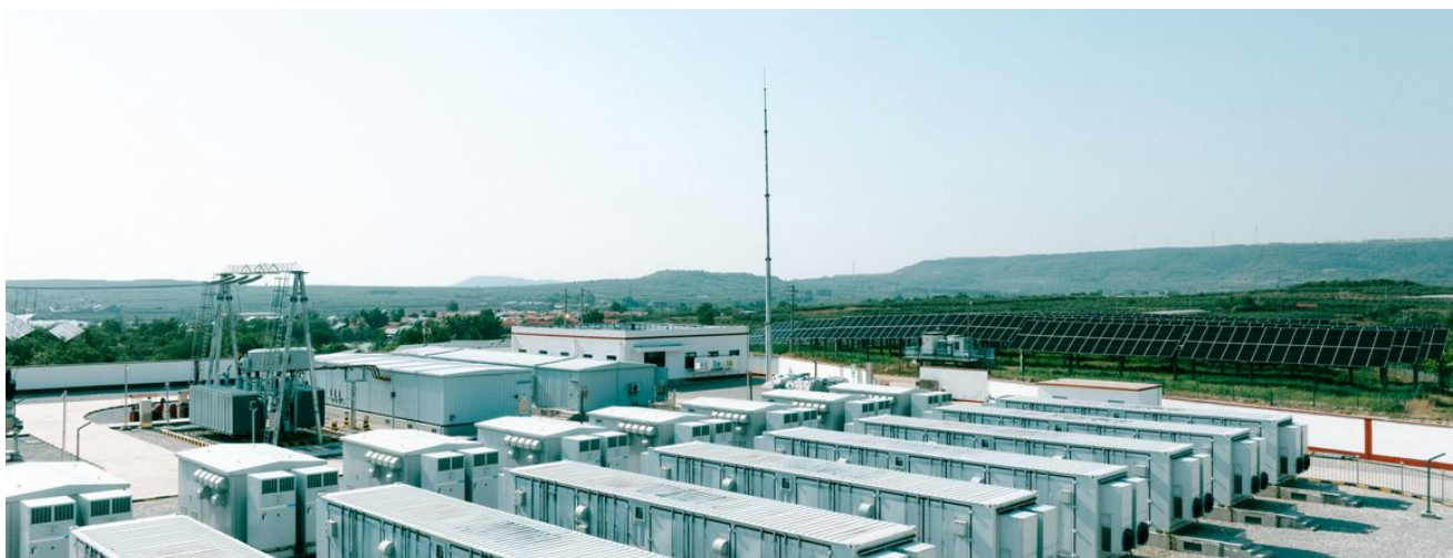
Battery storage, dispatched against a forecast.
